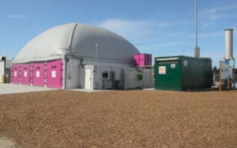
Equipment detail from ZWE's San Jose, California facility.
